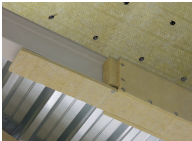
Fig. 15 The three side fire protection of a steel member in combination with the fire protection of a trapezoidal profile sheet. The thickness of the fire protection cladding ISOVER FireProtect® on the metal sheet corresponds to:
