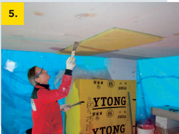
Press the first slab to the baseline and remove any excessive adhesive
