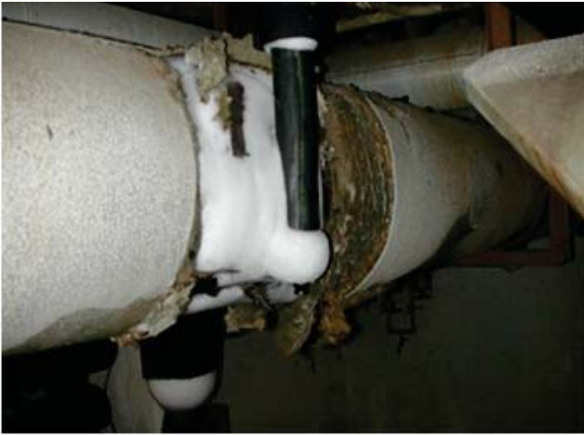
Figure 3: After cold services equipment has been in operation for a while condensation and eventually ice will form
