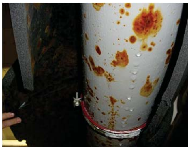
Figure 2: Consequences of not insulating pipe clamps on refrigeration pipes
